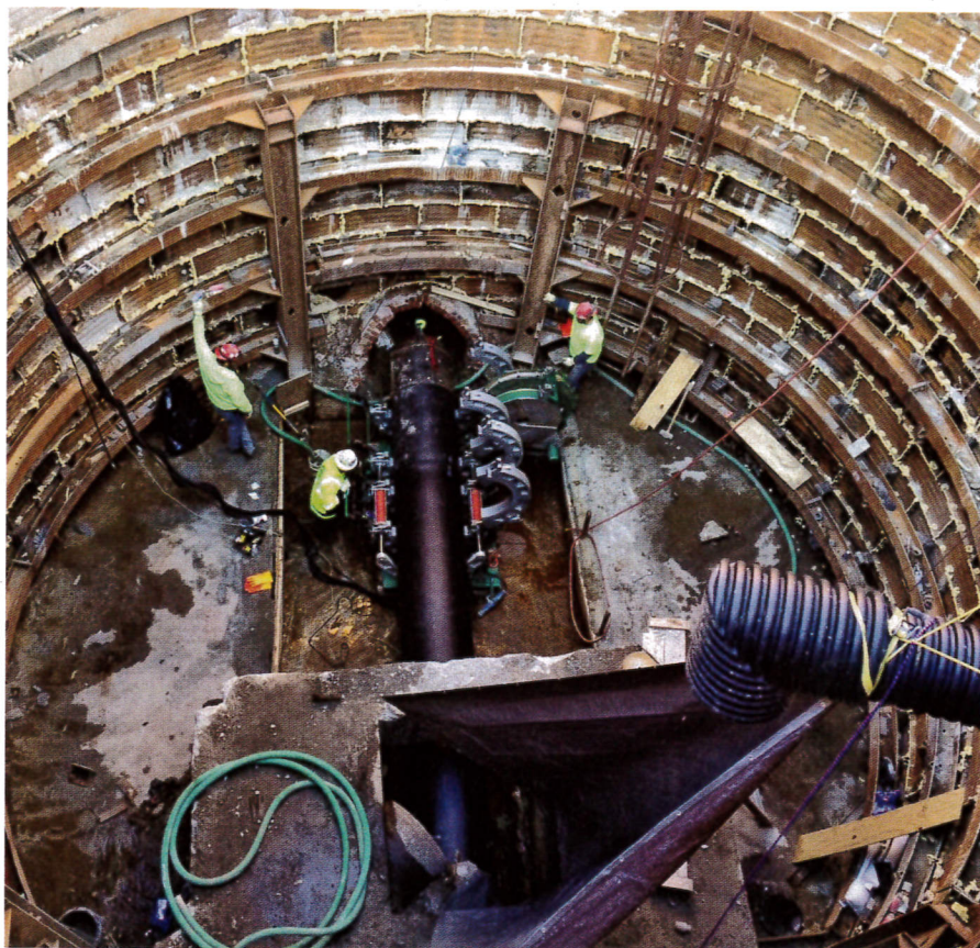
INSTALLING HDPE PIPE PROVED TO BE A WELL THOUGHT OUT AND WISE SOLUTION.
