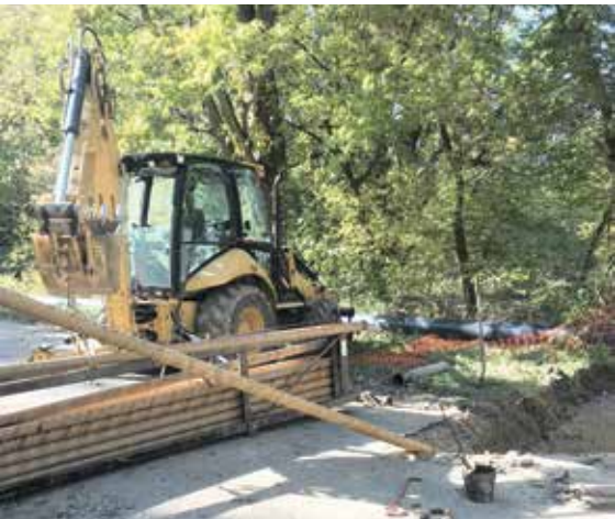
Took patience to work through cobble and hard consolidated clay under the river
